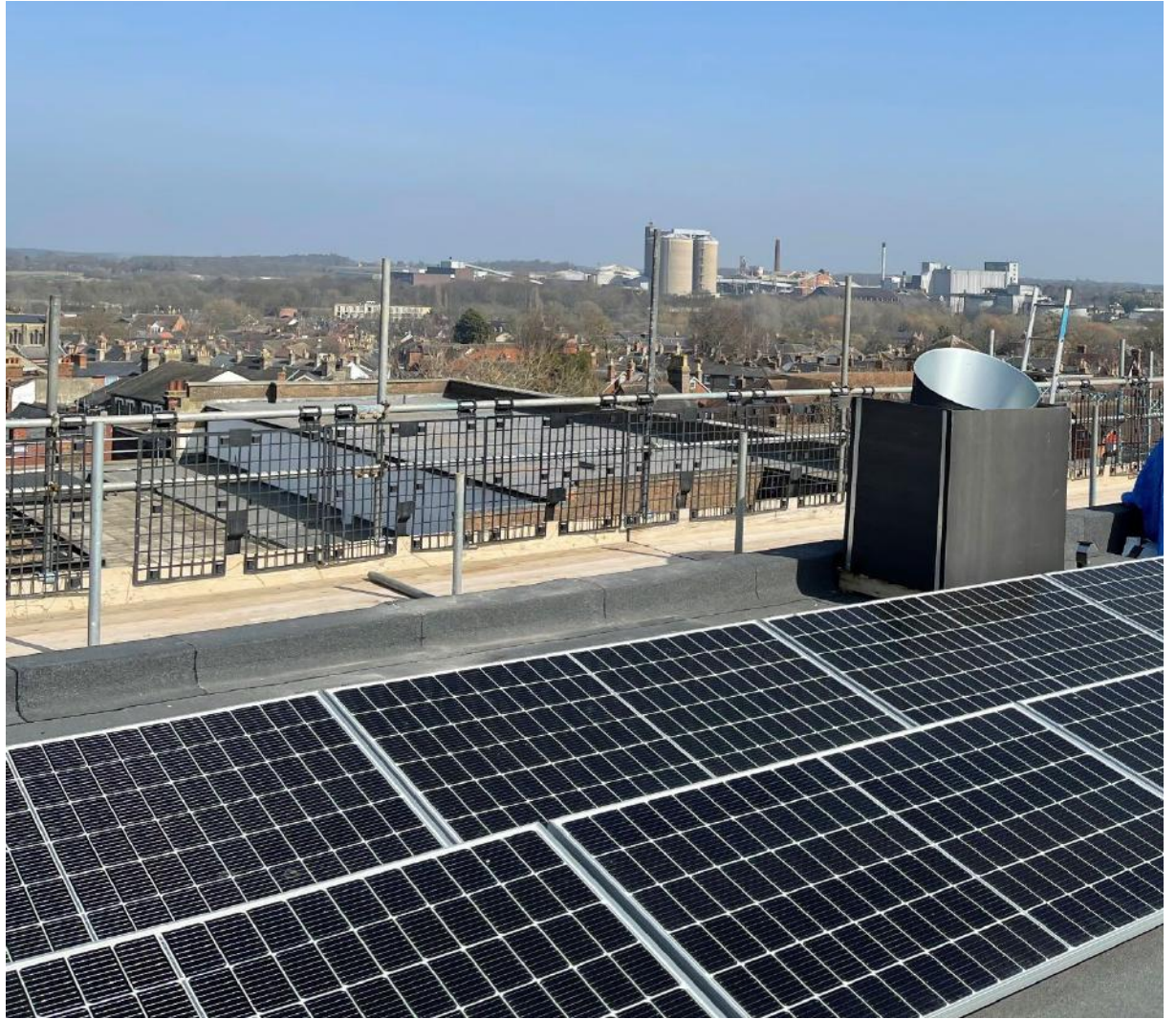
Image showing Photovoltaic panels at 17-18 Cornhill, Bury St Edmunds
